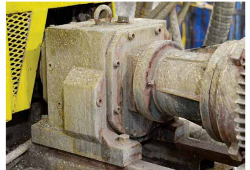
Lead Millwright Chris Stevens says he knows from experience that Dodge Quantis units are rugged and reliable. The proof, he says, is this Quantis ILH unit on a roll coater machine, one of the toughest applications in the mill. Despite the shock load and machine vibration, which has cracked the feet of other gearboxes, this Quantis reducer has performed without a problem for the past eight years.
